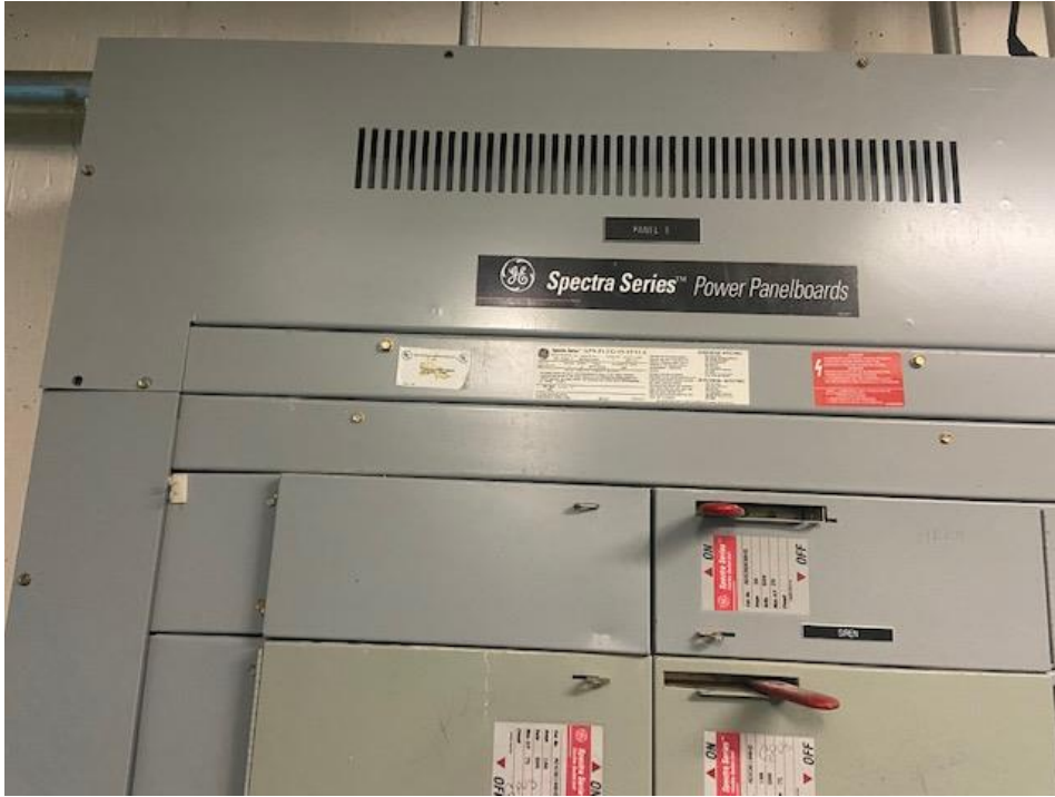
480 volt panel in basement of ARFF building to supply trailers.
