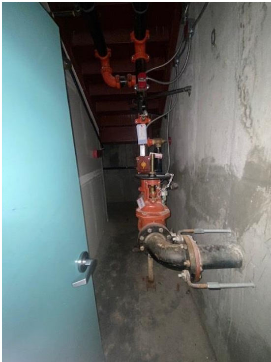
Utility entry point under stairway.
